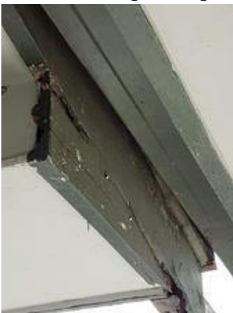
Photo of Workings/Damage
