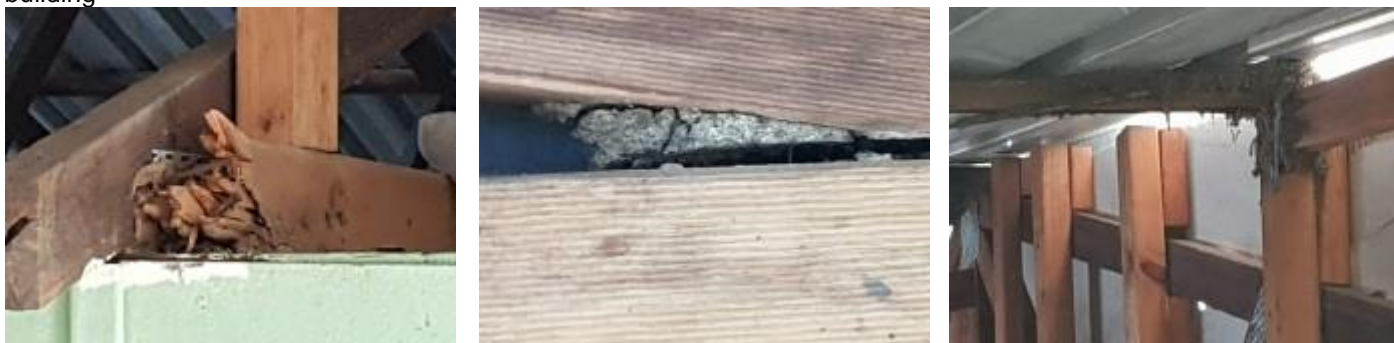
Extensive structural damage 2 old shed building
