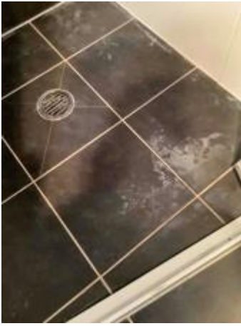
Discoloured Grout to Shower Floor
