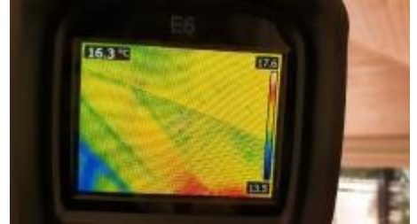
Thermal imaging did not pick up on any live termite activity to the structure at the time of inspection
