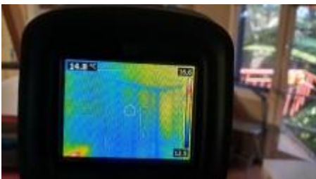
Thermal imaging did not pick up on any live termite activity to the structure at the time of inspection
