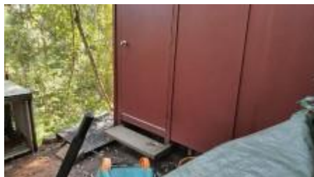
Carport/Shed is in direct contact with the ground and is conducive to termite activity and should be inspected on a regular basis for termite activity
