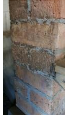
Very old workings located in subfloor/ workshop area.
