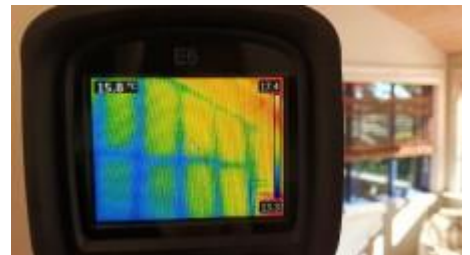
Thermal imaging did not pick up on any live termite activity to the structure at the time of inspection
