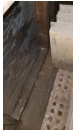
Lower level walls have no termite barriers and are installed directly onto the ground as seen from the subfloor areas, are conducive to termite activity and should be inspected on a regular basis
