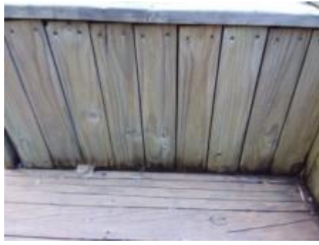
Slight woodrot and weathering to external timbers on decking areas
