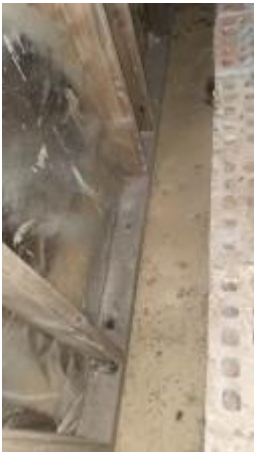
Lower level walls have no termite barriers and are installed directly onto the ground as seen from the subfloor areas, are conducive to termite activity and should be inspected on a regular basis
