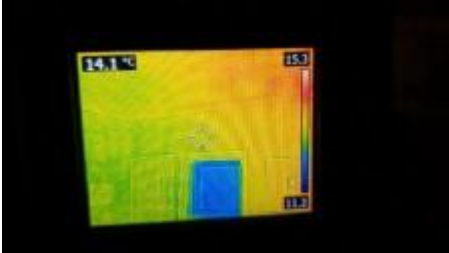
Thermal imaging did not pick up on any live termite activity to the structure at the time of inspection
