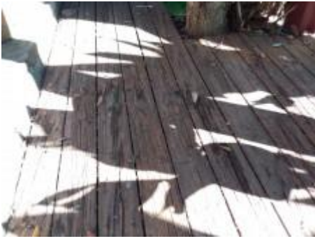
Weathering to decking areas
