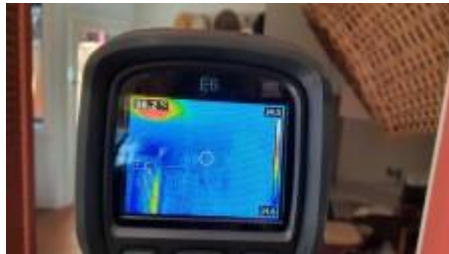
Thermal imaging did not pick up on any live termite activity to the structure at the time of inspection
