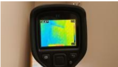
Thermal imaging did not pick up on any live termite activity to the structure at the time of inspection
