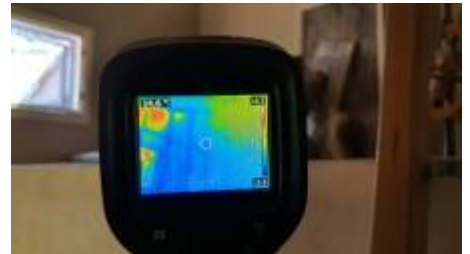
Thermal imaging did not pick up on any live termite activity to the structure at the time of inspection
