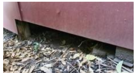
Carport/Shed is in direct contact with the ground and is conducive to termite activity and should be inspected on a regular basis for termite activity
